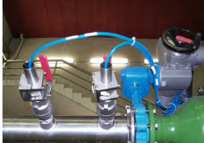
Nighttime supply flow measurement single path measurement in a full filled pipe
